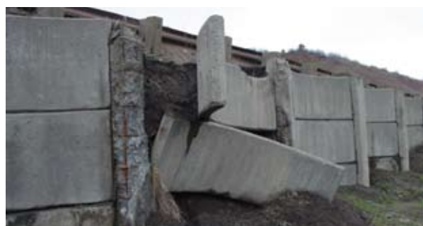
I-70 Wolcott – Safety Issues
