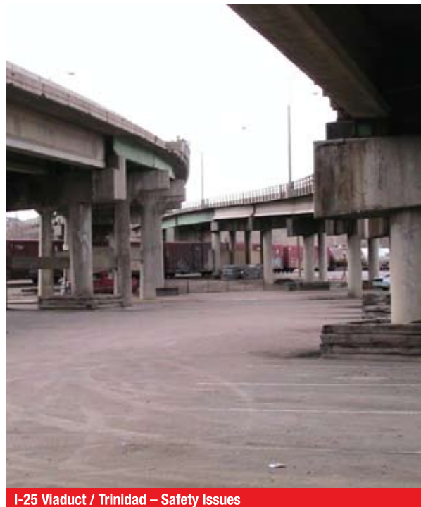
I-25 Viaduct / Trinidad – Safety Issues
