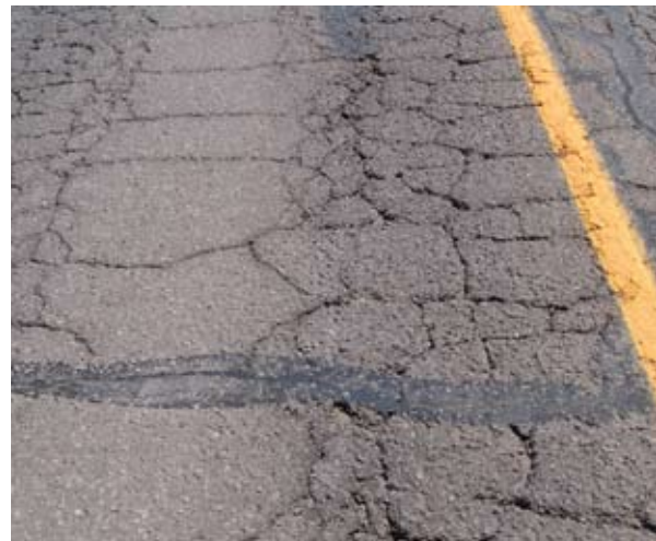
S.H. 141 – Surface Condition
