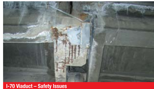
I-70 Viaduct – Safety Issues
