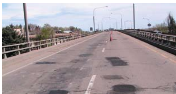
I-25 in Trinidad – Surface Condition
