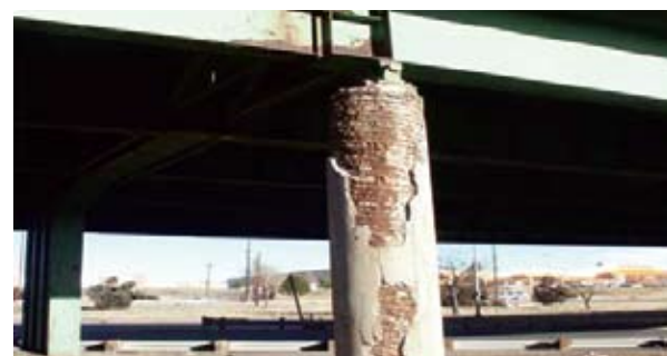
I-25 / Santa Fe Bridge – Safety Issues
