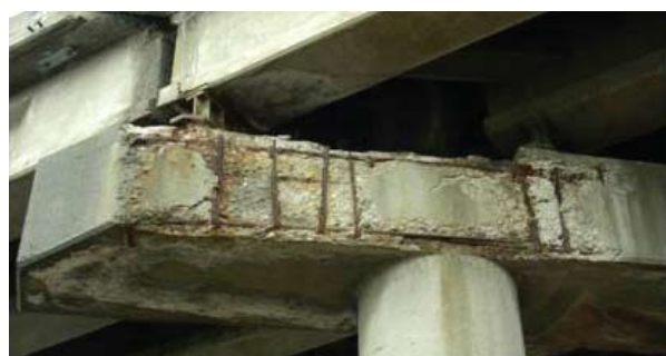
I-25 In Pueblo – Safety Issues
