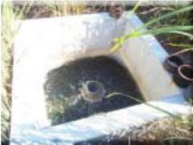
Removable sleeves are used to control the water elevation in the wetland cells.
