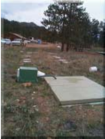
Septic tank system
