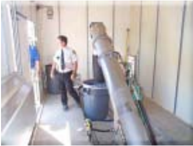
Mechanical fine screen (ROTOMAT) headworks facility
