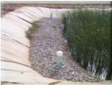
Buried inlet pipe with stub-outs for maintenance
