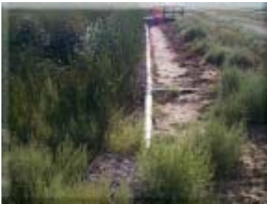
Influent pipe to wetland
