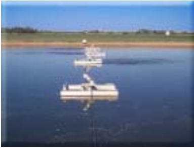
Aerators on lagoon
