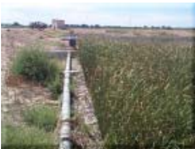
Influent pipe to cell #1
