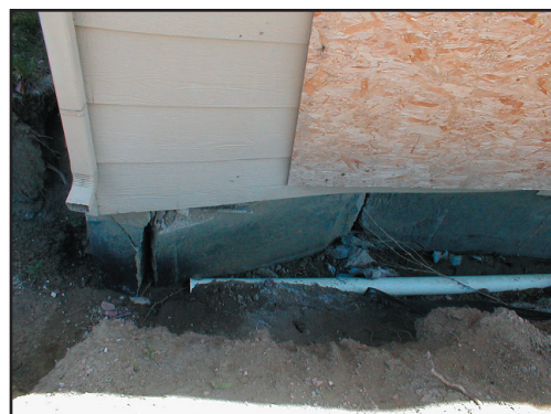
Landslide Damage to Home in Colorado Springs Photo provided by Colorado Springs OEM
