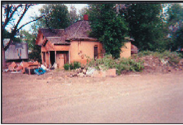
Home flooded in Otero County in 1999, Photo provided by the Colorado Water Conservation Board
