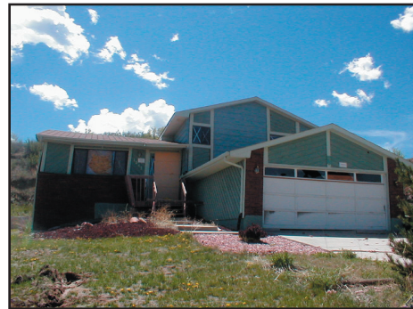
Home Destroyed by Landslide in Colorado Springs Photo provided by Colorado Springs OEM
