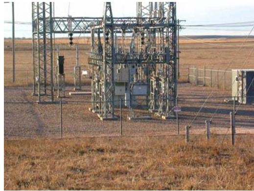
Typical HEA Distribution Substation
