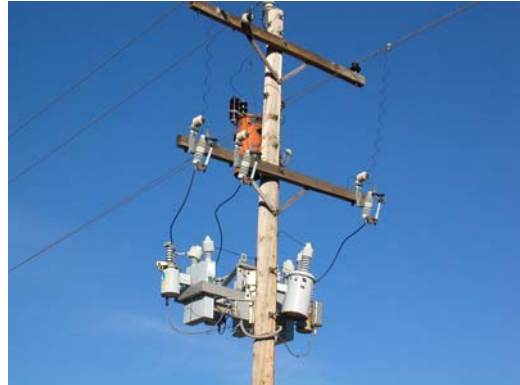
Three-Phase Capacitor Bank
