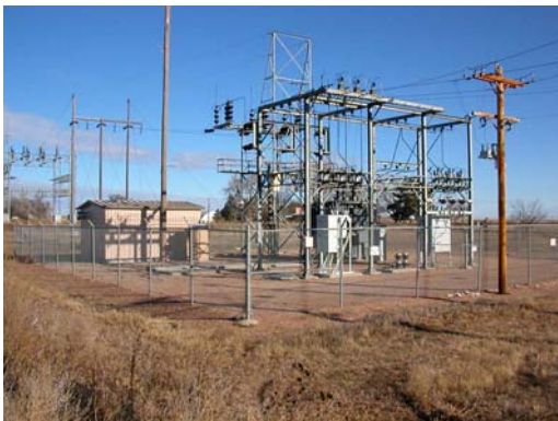
Julesburg Distribution Substation
