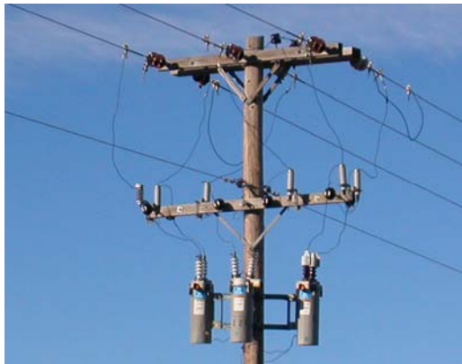
Three Single-Phase Reclosers
