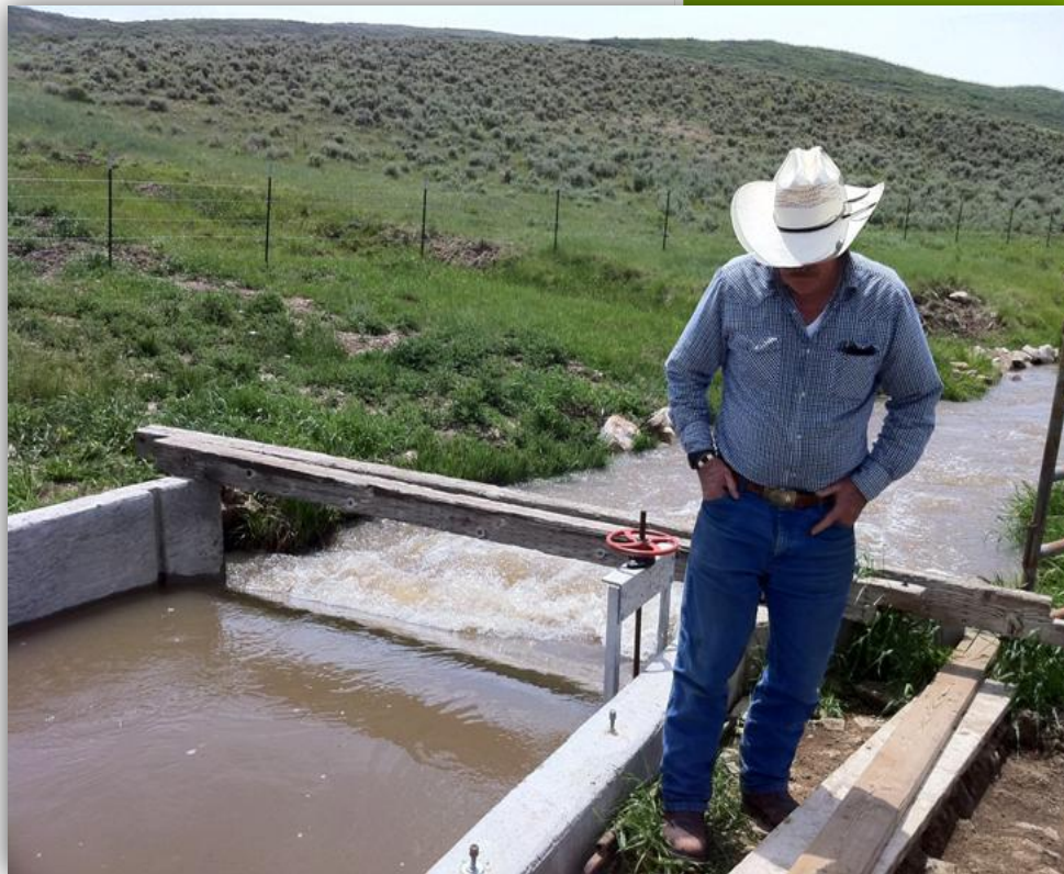
23 kW hydropower utilizing an existing irrigation ditch in Meeker, Colorado
