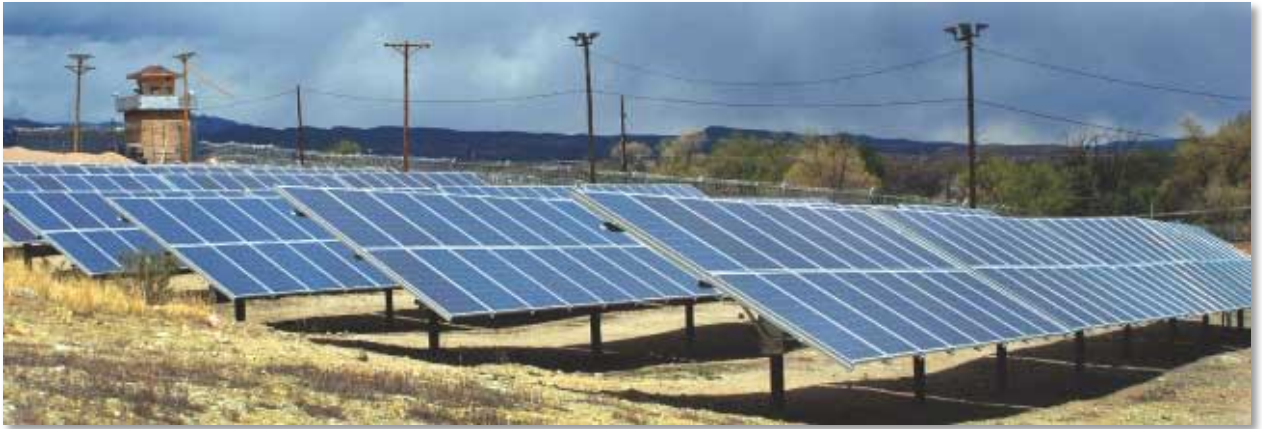
Figure 1. Solar panels recently installed at Colorado Territorial prison in Canon City
