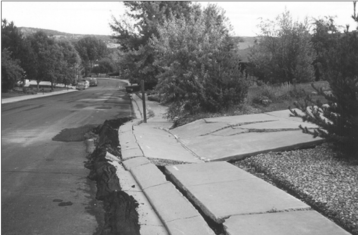
Figure 12. Damage to Hofstead Terrace roadway pavement, sidewalk, and driveway by lateral movement of landslide toe at Hofstead Landslide in 1999. Photo by J. White.
