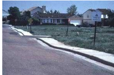
Expanding soils buckle many roads in Colorado. Image from the Colorado Geological Society
