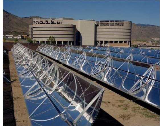
Solar Thermal Collector System Thermal collectors capture solar energy and convert to heat, which is then utilized directly, or converted to electricity. Pictured: A medium temperature parabolic trough solar thermal collector system provides for facility and water heating at Jefferson County Detention Center in Golden, CO. Image: NREL, 2011
