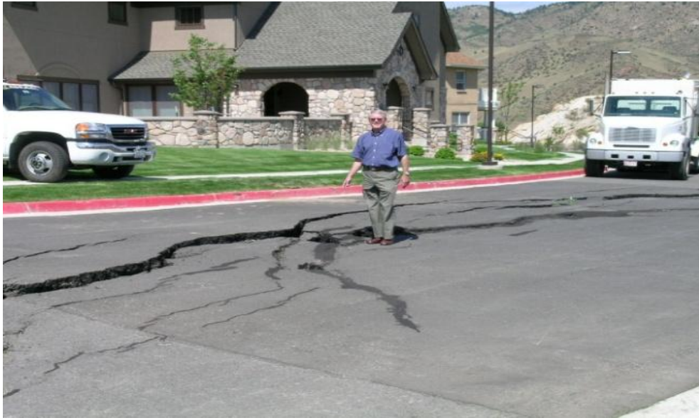
A buckling road in Golden, Colorado; photo by TC Wait
