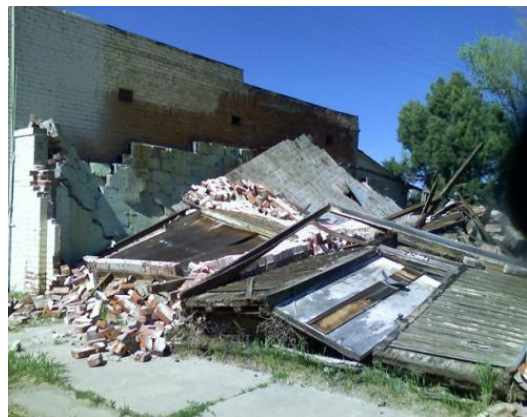
High winds are responsible for toppling this structure next to the Agate Post Office in Elbert County in 2010
