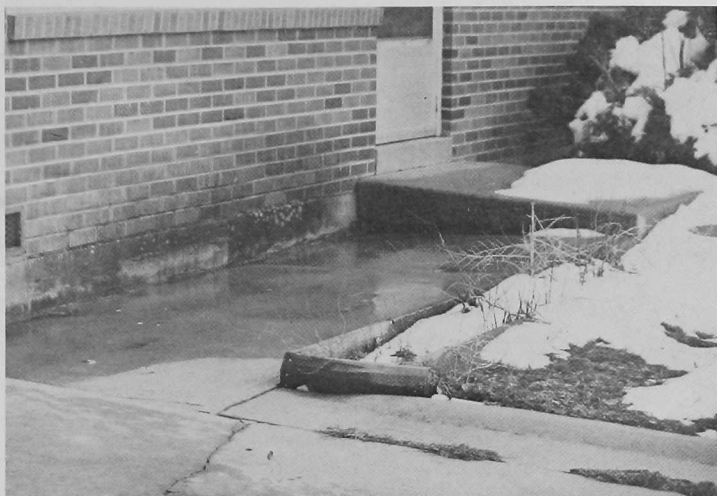
Figure 27. Settlement of the fill material has resulted in reversed drainage next to the foundation.
