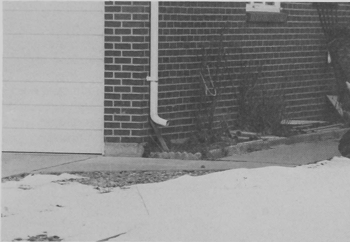
Figure 22. People often remove the downspout extension so that their flower bed can be watered by storm runoff.
