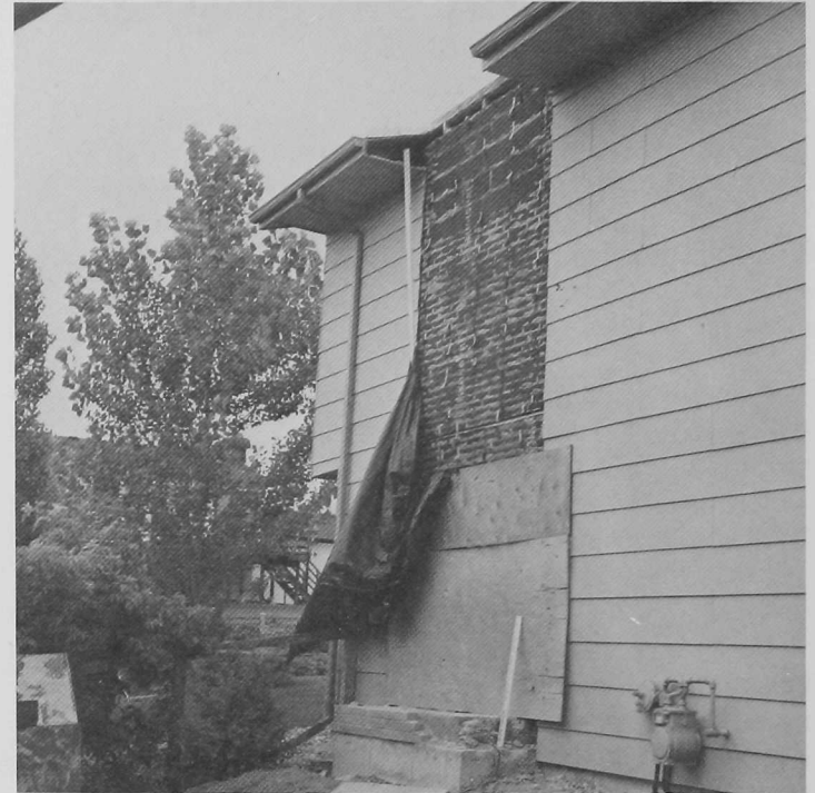
Figure 32. The chimney of this house located in a southwest Denver suburb separated from the house and had to be removed before it collapsed. It was damaged by swelling soils.
