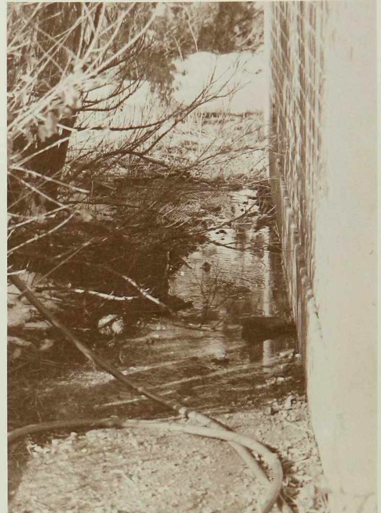
Figure 13. The lack of gutters on this house has allowed snowmelt to run over the eaves and pond next to the foundation.
