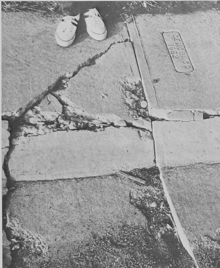
Figure 31. Swelling soil is responsible for the destruction of this sidewalk.
