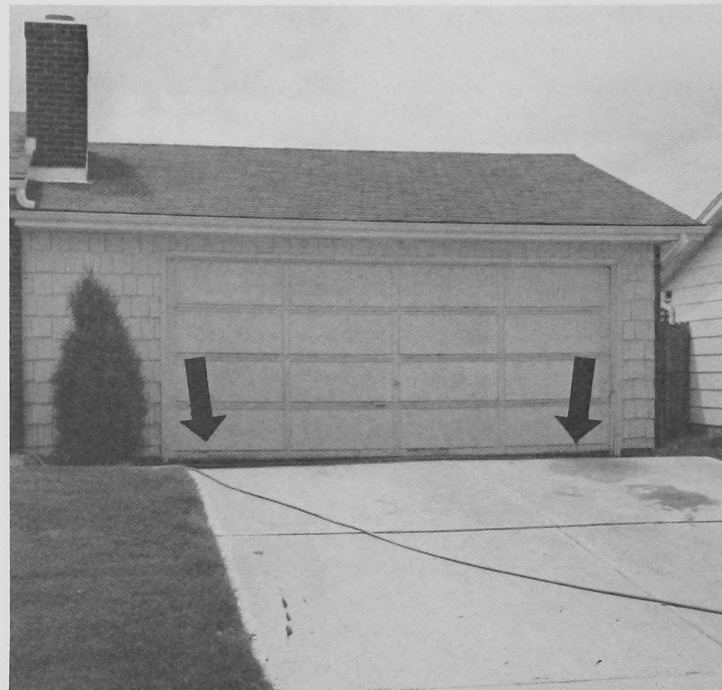
Figure 30. Swelling soil has caused this driveway to heave. Note the gaps where the garage door meets the driveway.
