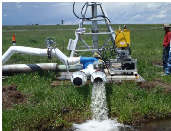
Figure 14: Bear River Ranch turbine
