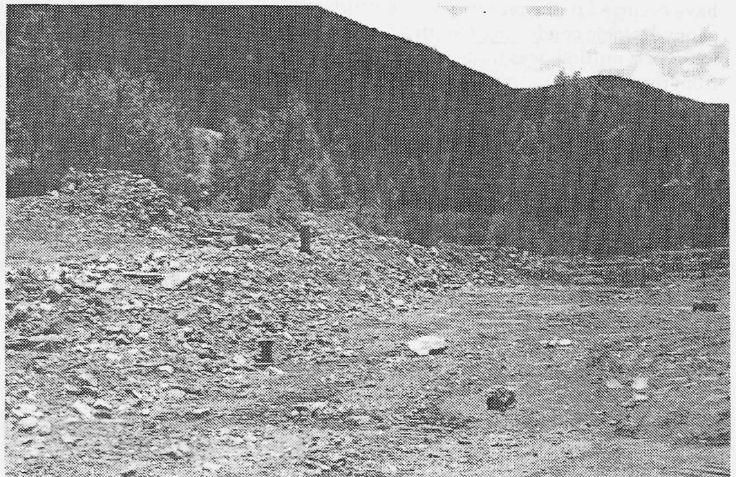
Figure 7. Water line on flooded bench. The riser pipe in the lower foreground and the hydrant are connected to the water line.
