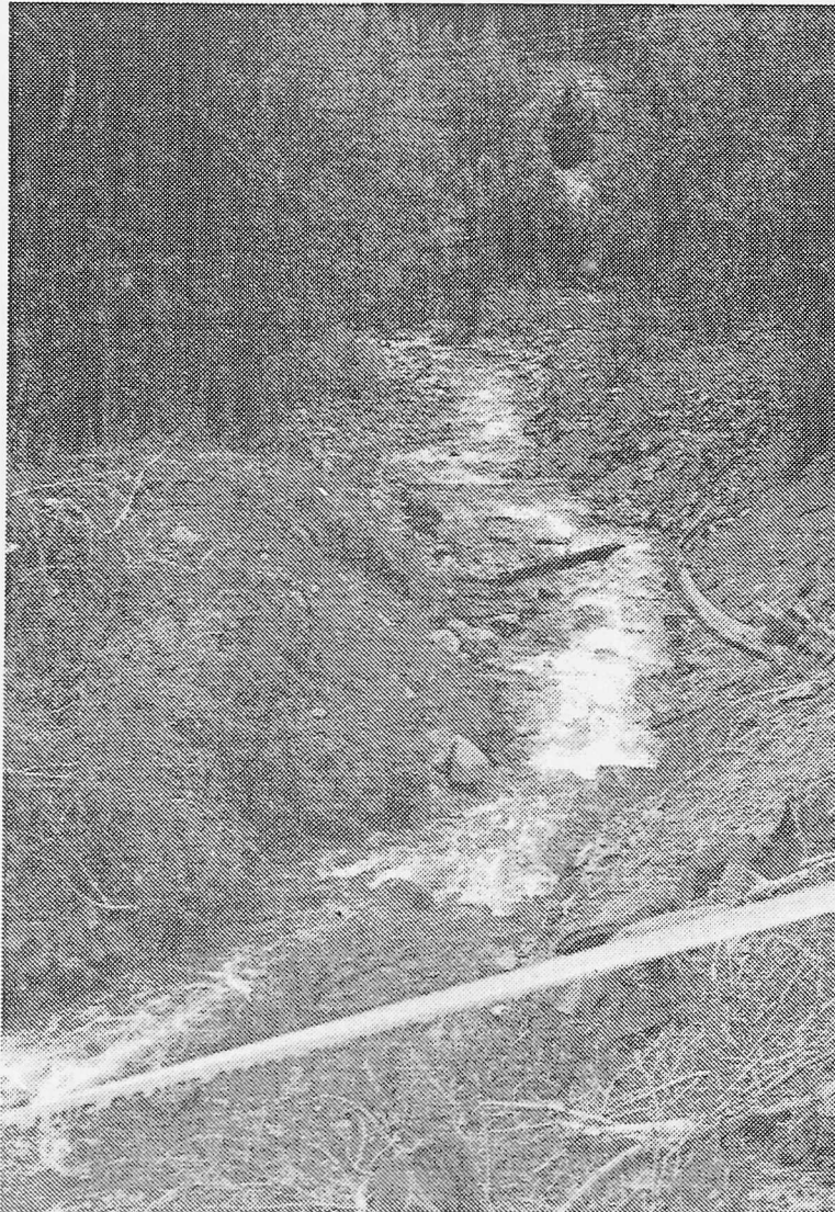
Figure 4. Location of whirlpool and cribbing encountered during re-alignment of Silver Creek channel. The loose fill material on the left side of the Creek in the center of the picture was dumped into the whirlpool.
