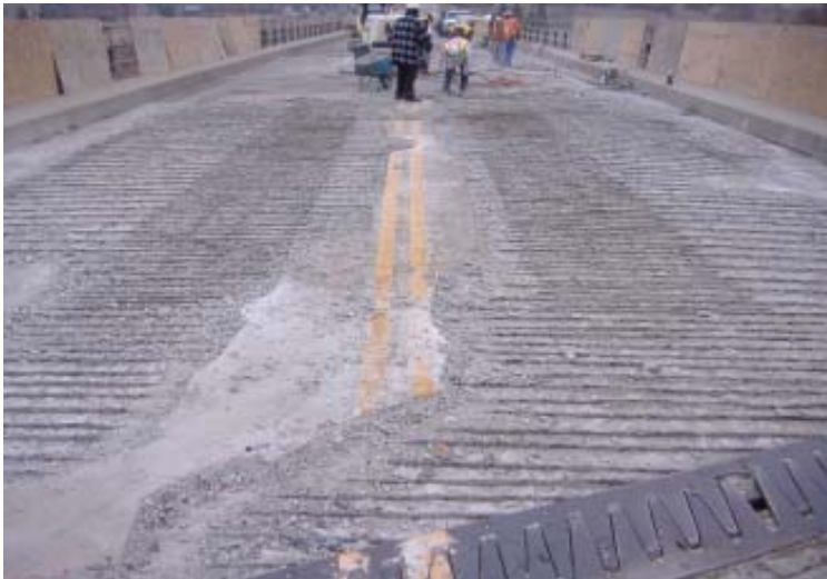
Bridge deck rehabilitation is underway on the Tabor Street bridge over I-70 (Project #15).
