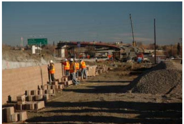
Crews construct a retaining wall near the new flyover from eastbound I-70 to westbound SH 58 (Project #10).
