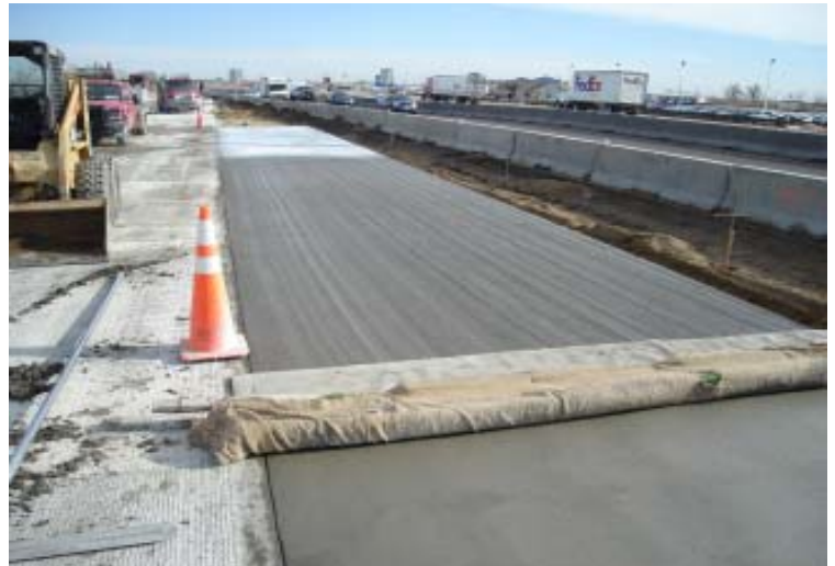
Concrete paving of some new I-25 lanes is underway as part of the I-25 widening project between SH 52 and SH 119 (Project #33).
