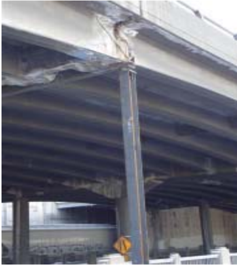
Current condition of expansion joints on the I-70 viaduct (Project #11).
