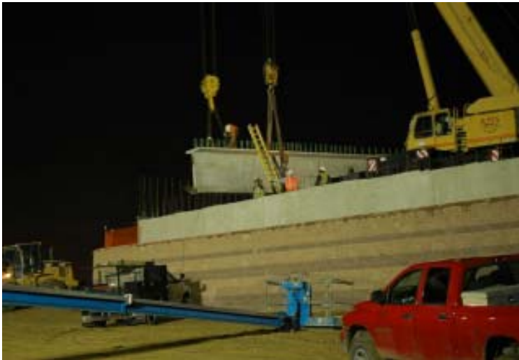
Crews install girders for the new 128th Avenue bridge over I-25 which will carry four lanes instead of two (Project #3).
