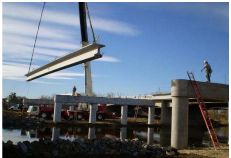
Crews install girders for the new I-25 bridge over the St. Vrain River as part of the I-25 widening project between SH 119 and SH 66 (Project #34).
