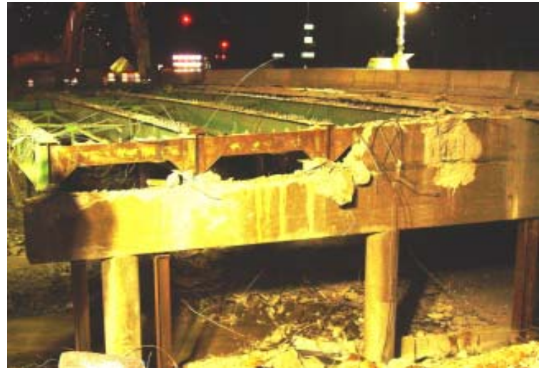
The eastern portion of the existing Washington Avenue bridge over SH 58 is demolished (Project #8).
