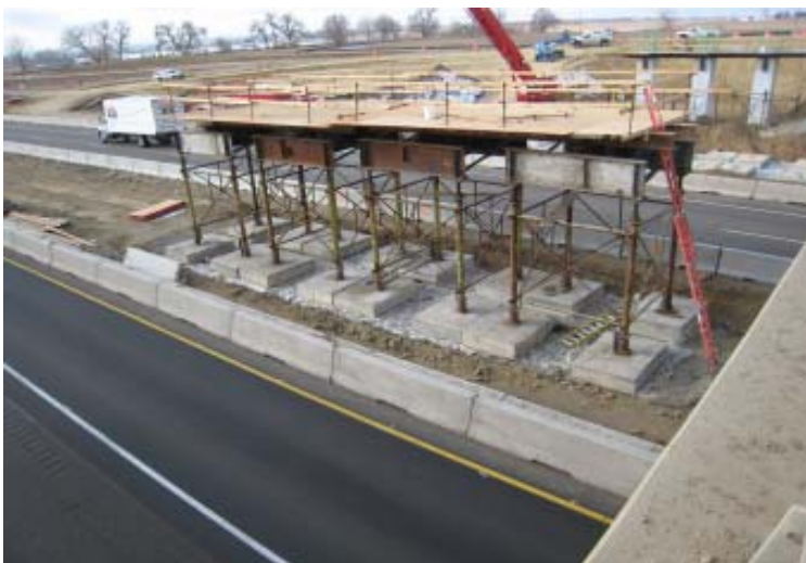
The new SH 66 bridge over I-25 under construction as part of the I-25 widening project between SH 119 and SH 66 (Project #34).
