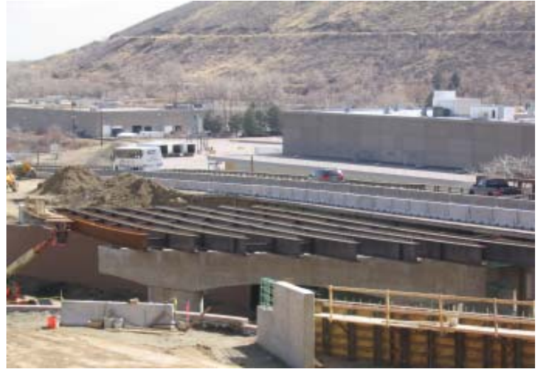
Girders have been installed for the new westbound SH 58 bridge over 44th Avenue (#12).
