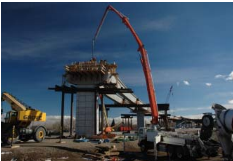
Construction of the new flyover from eastbound I-70 to westbound SH 58 (Project #10).
