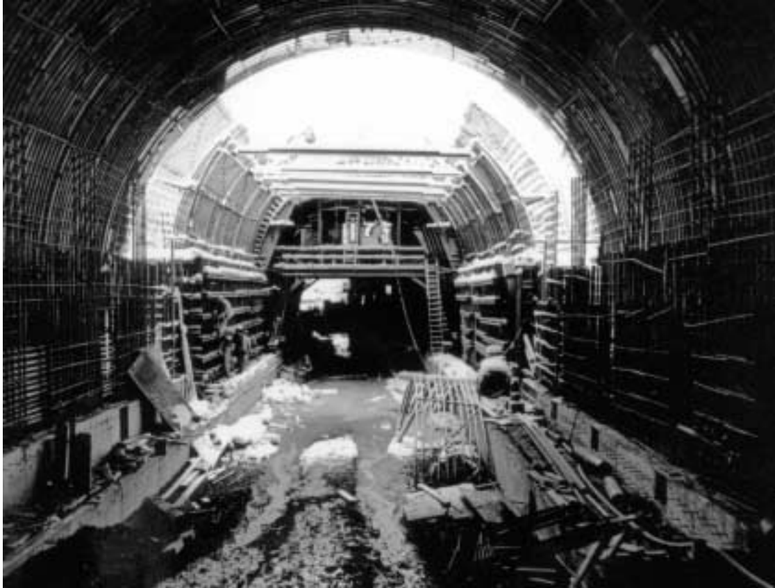
Plate 7. Perhaps the greatest engineering accomplishment in state history, the Eisenhower Tunnel took 13 years and $125 million to complete. Vital to the completion of Interstate 70 through the Continental Divide, the tunnel linked for the first time the eastern and western halves of Colorado. Source: Denver Public Library – Western History Department © 1995-2002 Denver Public Library.
