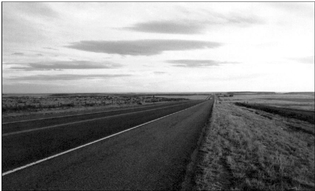
Plate 33. Steep embankments on both sides of US 385 southwest of Lamar near the local airport.
