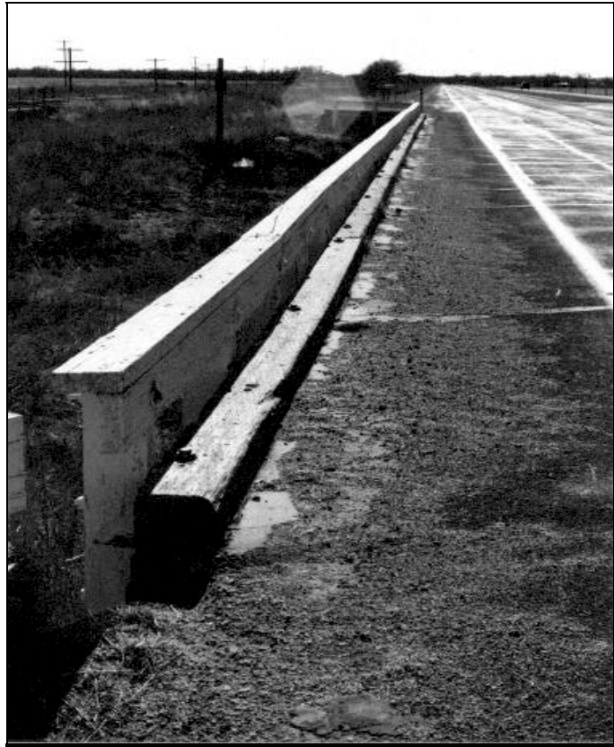
Plate 18. Timber curbing along bridge over Pawnee Creek, Logan County. View south down US 6.
