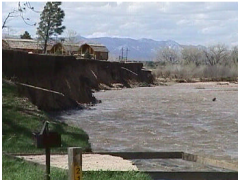
Damage to KOA campground along Fountain Creek south of Colorado Springs.
