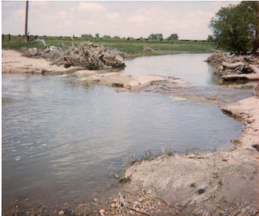
WCR 67 at Crow Creek. Road washout and debris deposition.
