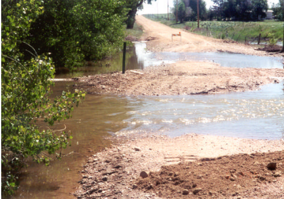
Road surface damage on WCR 74 from Crow Creek floodwaters between WCR 392 and 79.
