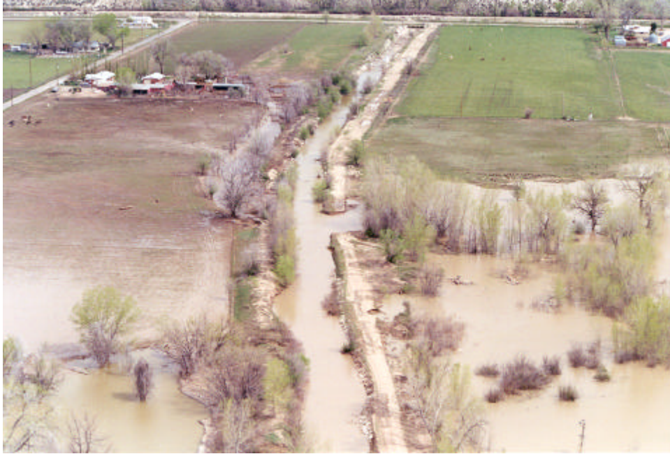
Break in the Fort Lyon Sluice #2 (Fort Lyon Canal in background). May 3, 1999
