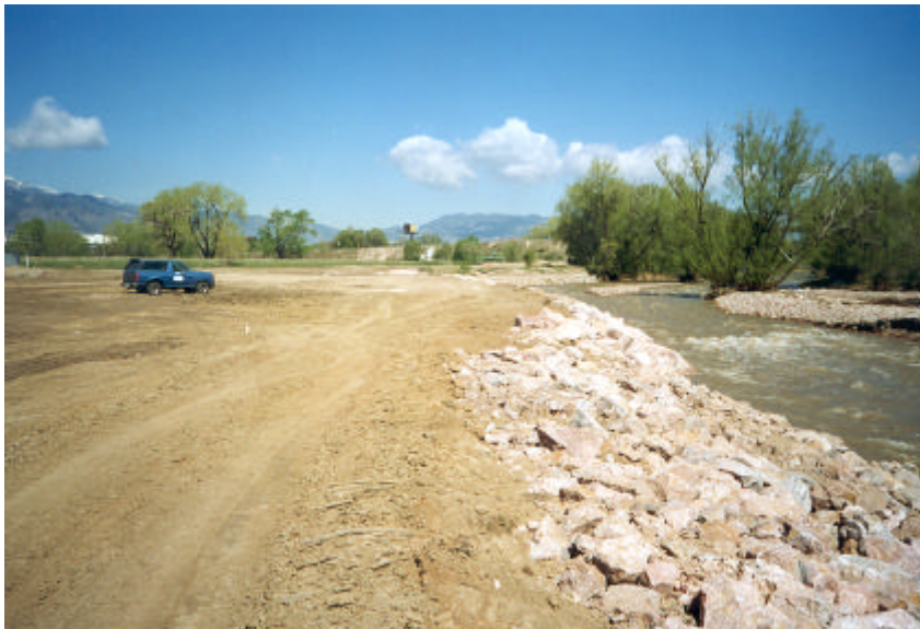
Emergency work to repair 48-inch interceptor south of Circle Drive and east of Janatell Road after completion.
