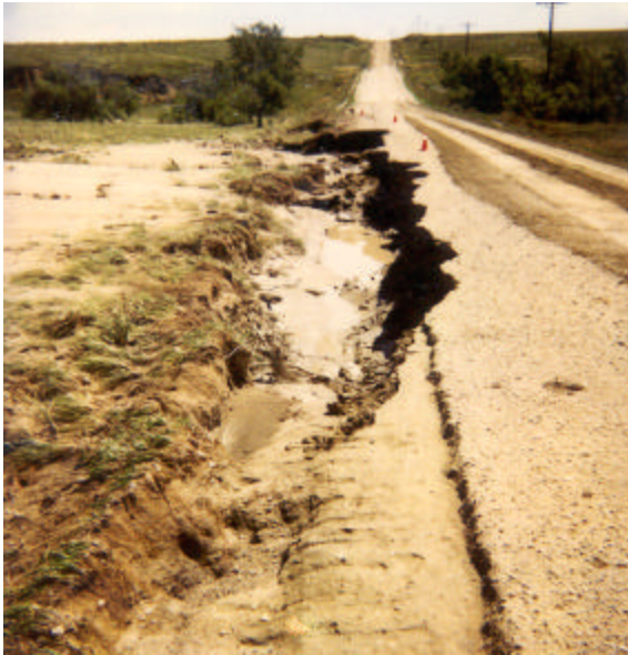
Washout on CR 154 caused by flood waters in Middle Bijou Creek.
