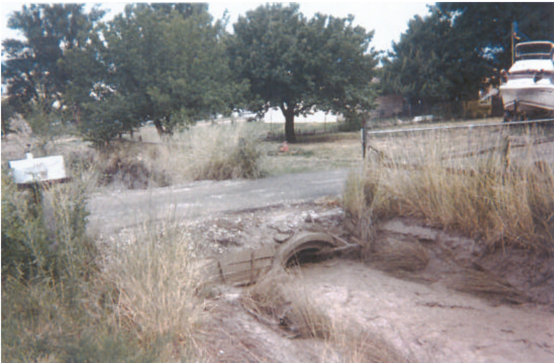
Bosley Wash 48-inch culvert at 3445 F \frac{3}{4} Road (1999 storm event).
