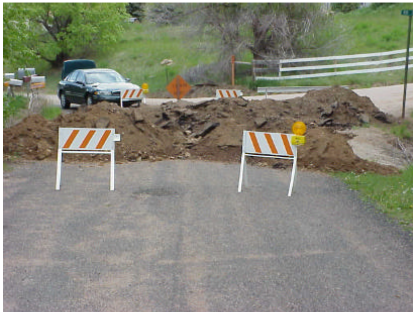
Washed out County Road 389 crossing.
