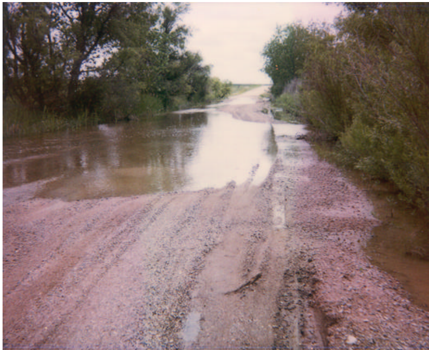
WCR 110 between US 85 and WCR 27 where floodwaters from Lone Tree Creek overtopped the road for 755 feet.
