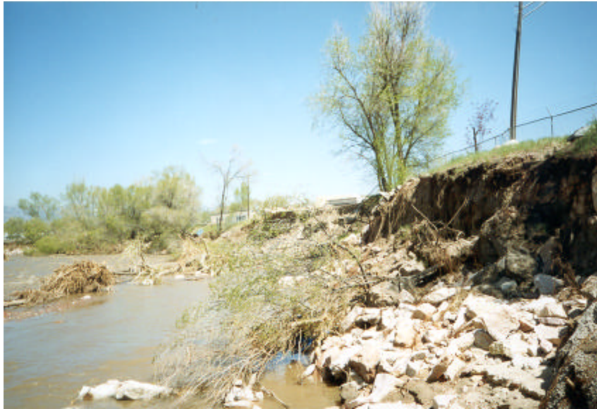
Fountain Creek erosion adjacent to the Las Vegas Street Wastewater Treatment Plant.
