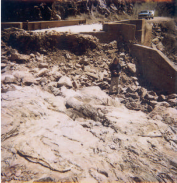
Damage to County Road 67, Phantom Canyon.
