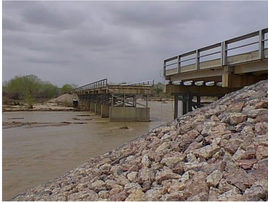
Piñon Bridge over Fountain Creek looking west after the flood.
