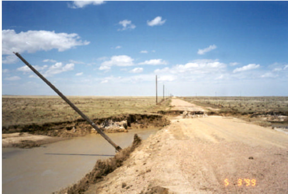
Wash out on Lane 21 just north of a bridge over Breckenridge Creek.
