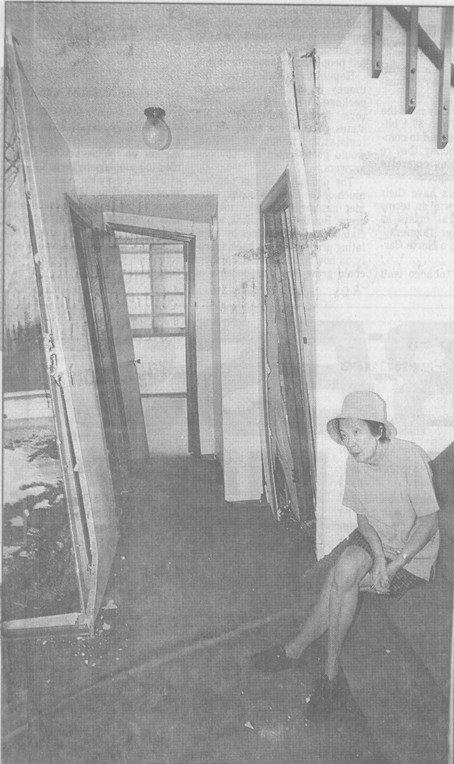
Netta Lowderman sits on steps leading to the family room, where walls have shifted and cracked. Her house has been condemned.
