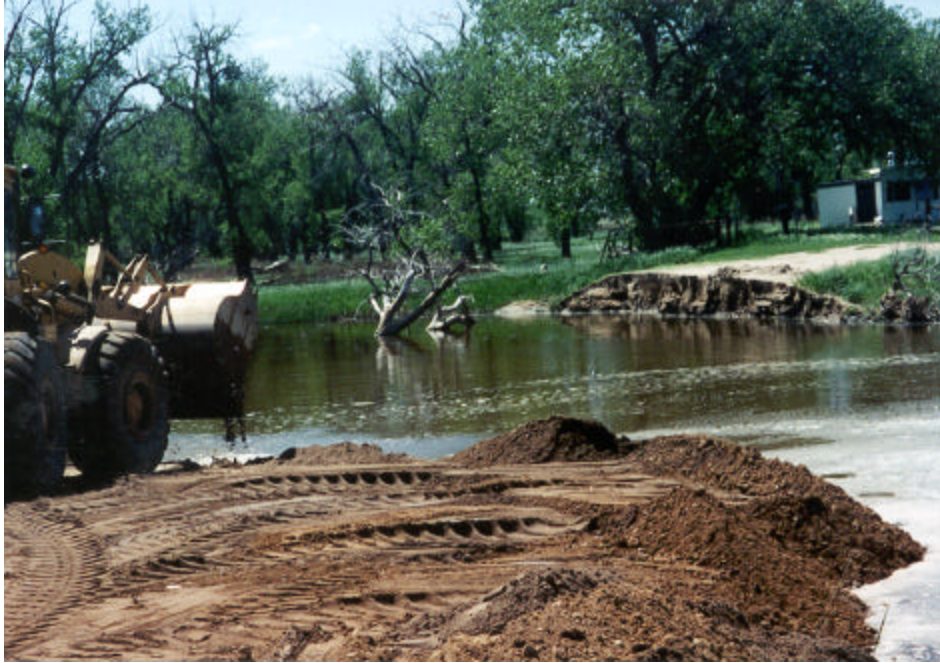
Repair work at the WCR 87 crossing of the Poudre River between WCR 42.5 and 44.5.
