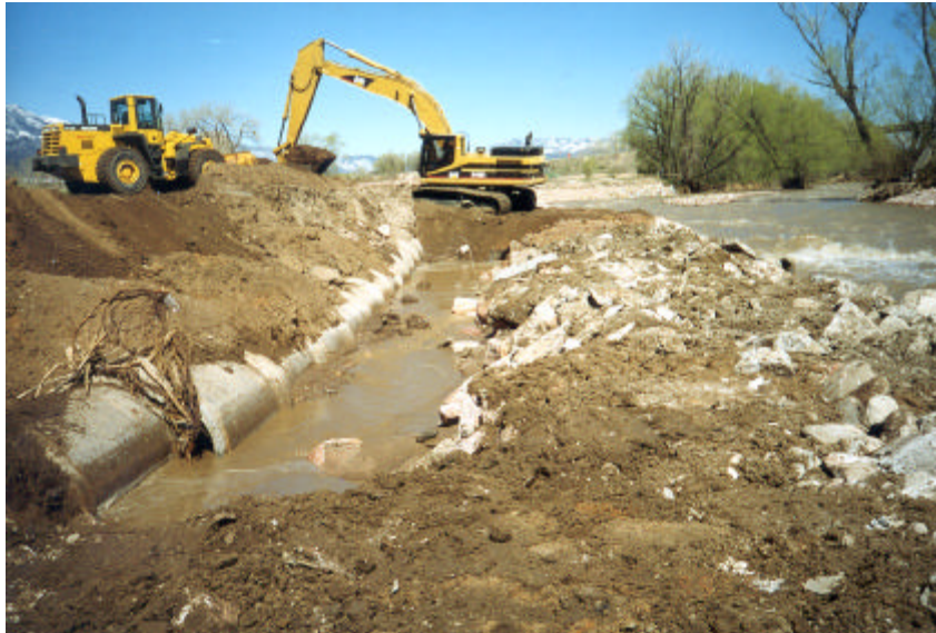
Emergency work to repair the 48-inch interceptor and stabilize Fountain Creek bank. Location is south of Circle Drive and east of Janatell Road.
