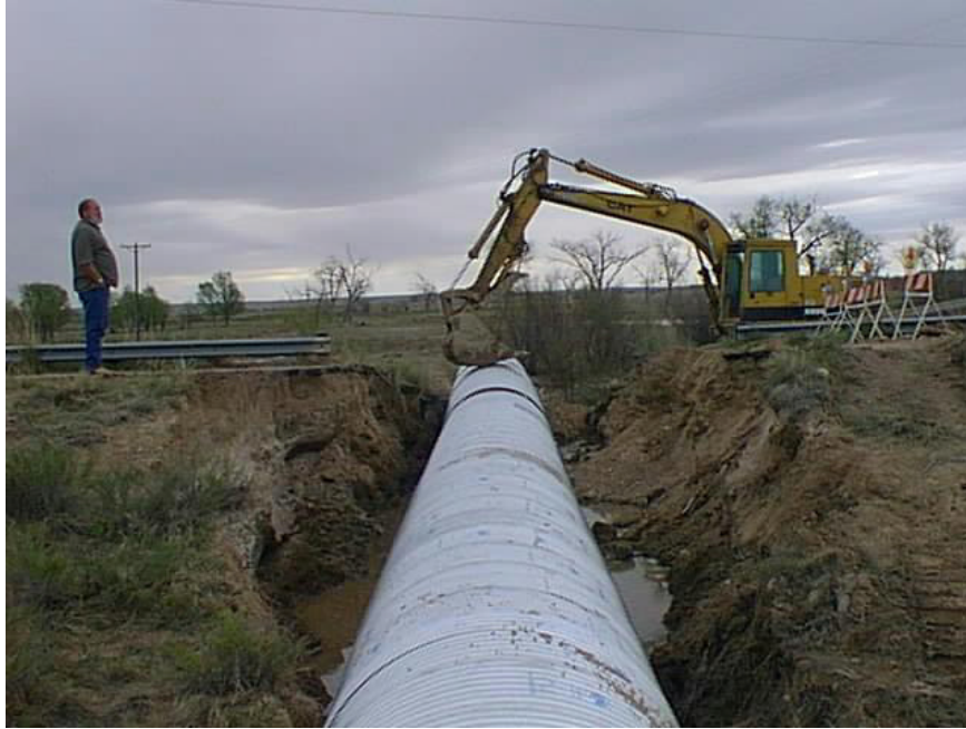
Replacing washed out culvert under C-209, south of Boone on north side of Arkansas River.
