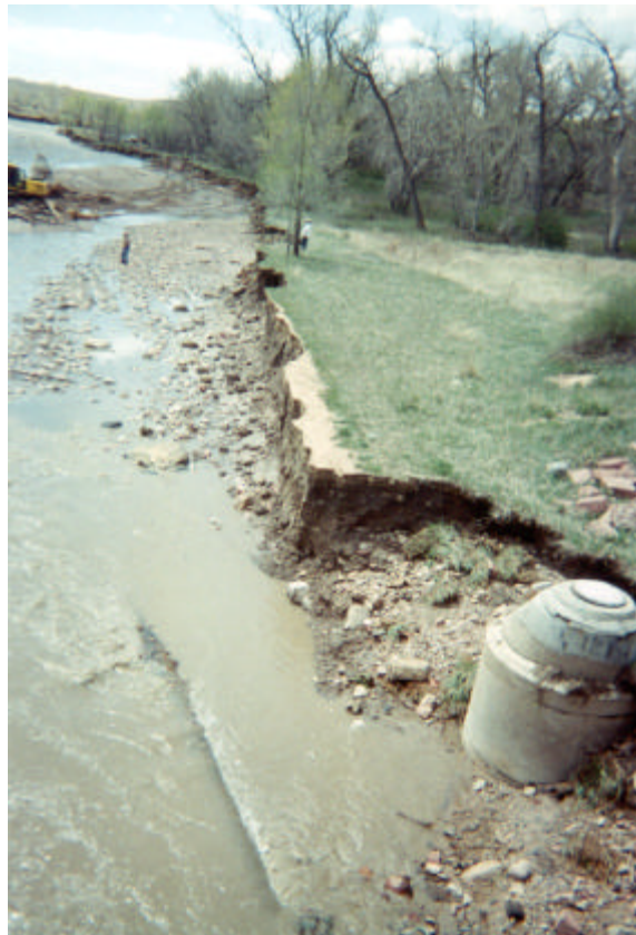
Erosion along Fountain Creek exposed 30-inch sanitary sewer force main and eventually ruptured the line.
