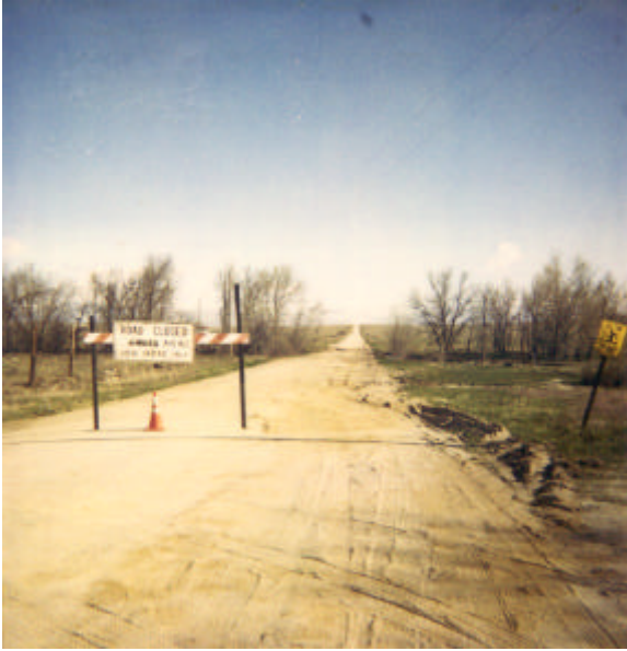
County Road 149 near the town of Matheson closed due to a washout.
