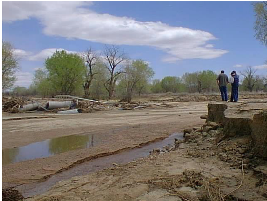
Former west approach to Piñon Bridge looking east (note washed out 72-inch culverts).
