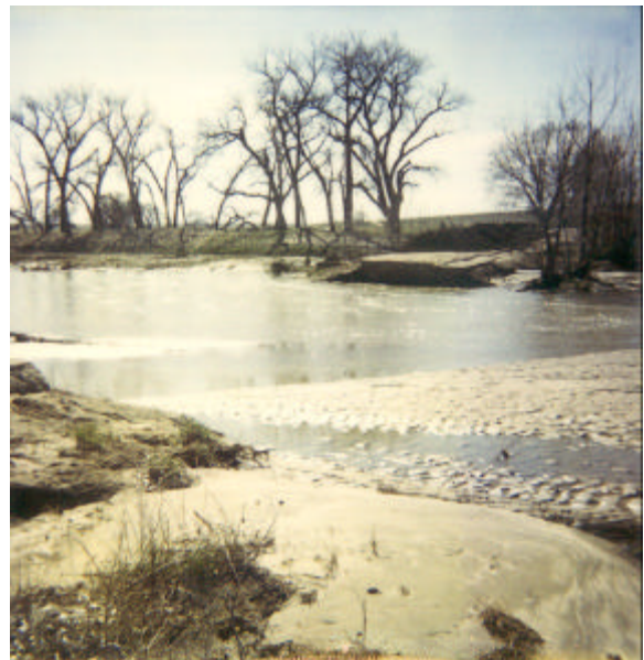
CR 118 west end washed out by flood waters in Big Sandy Creek.
