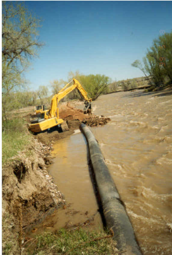
Emergency work to rebury the 30-inch sanitary sewer south of Circle Drive and stabilize the creek bank.
