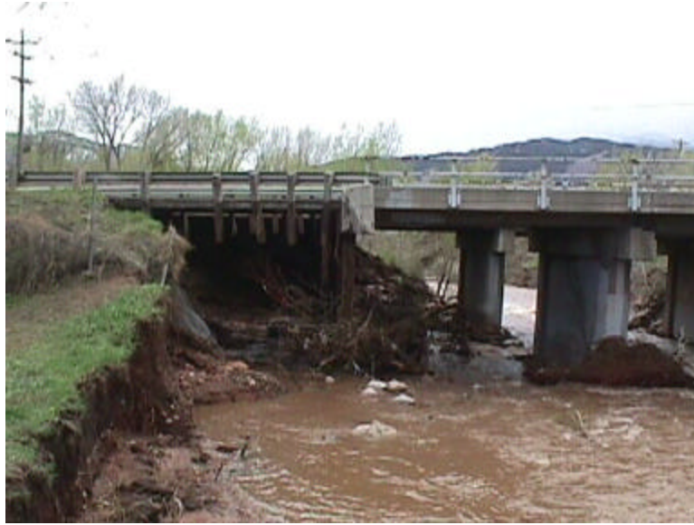
Highway 24 bridge abutment washout on Fountain Creek upstream of Colorado Springs.
