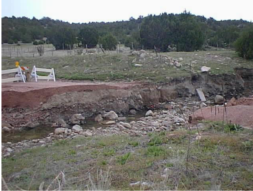
Washed out culvert and road crossing on Red Creek Springs Road.
