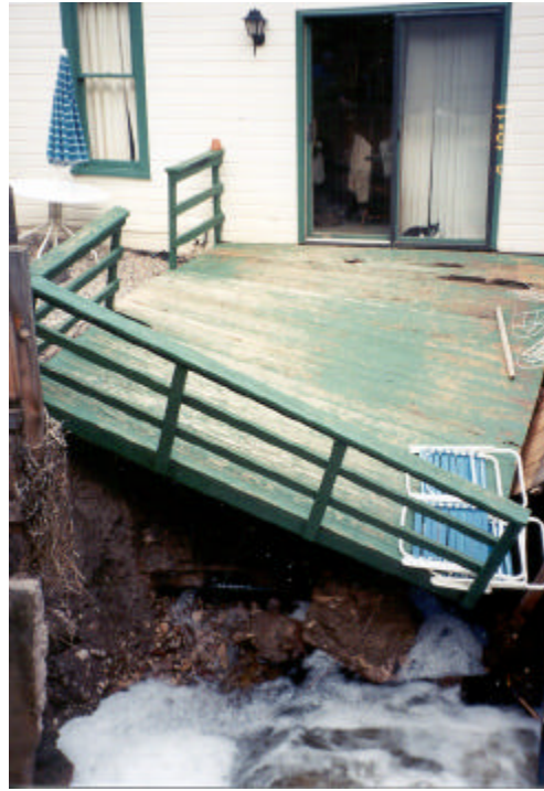
Deck lost to erosion along Williams Canyon in Manitou Springs.
