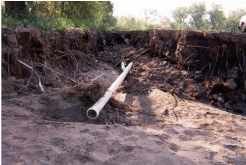
Damaged to pressurized sewer line at the BSD facility.
