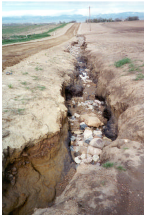
Borrow ditch on WCR 30 between US 85 and WCR 31 eroded by local runoff to a depth of 4 feet.
