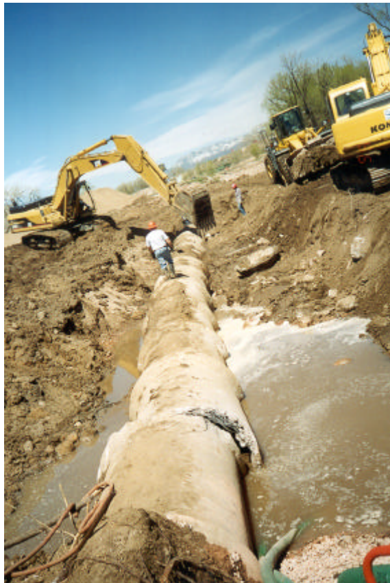
Ruptured 48-inch sanitary sewer interceptor along Fountain Creek.
