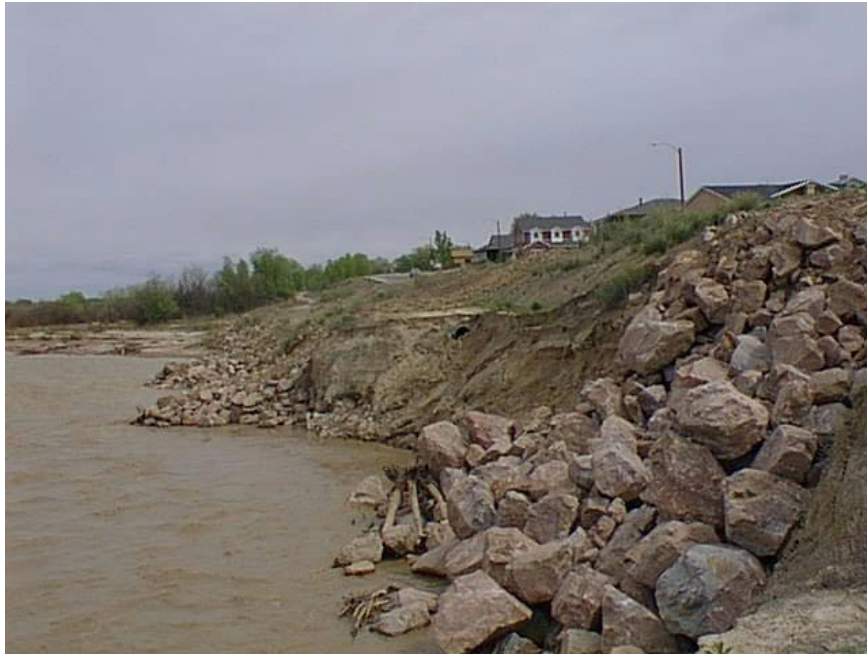
Chinook Lane at Fountain Creek in Pueblo looking upstream (bike path and sanitary sewer line washed out, large riprap placed later to hold remaining bank).
