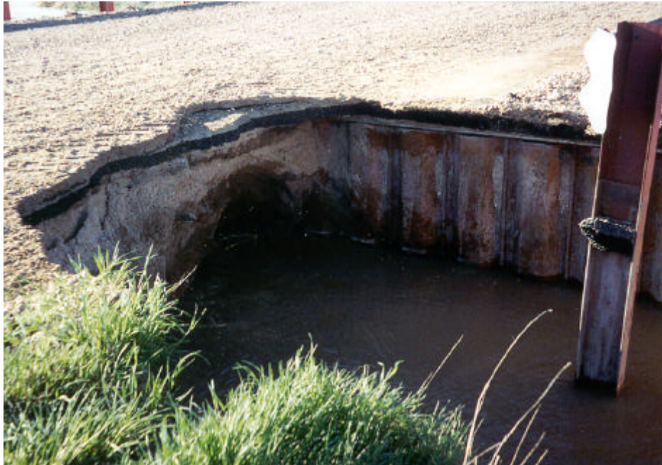
Crow Creek scoured out a 30' W × 10' L × 8' D hole behind a bridge wing wall on WCR 83 between WCR 94 and 100.
