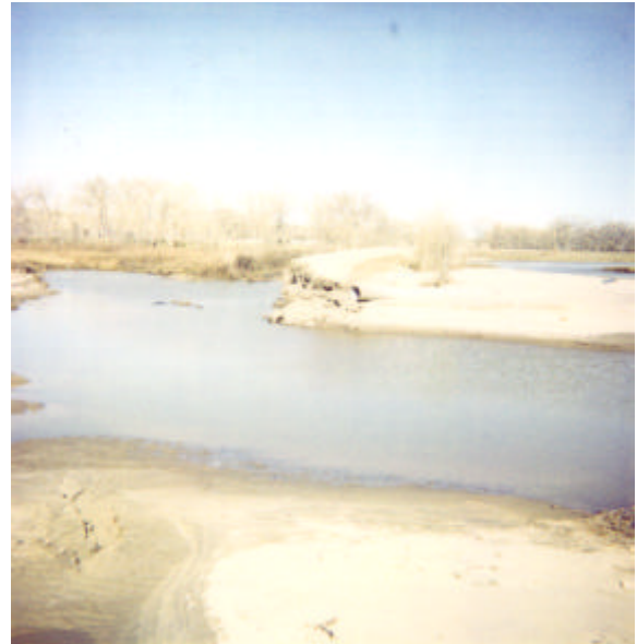
CR 118 east end was damaged by flood waters from Big Sandy Creek.
