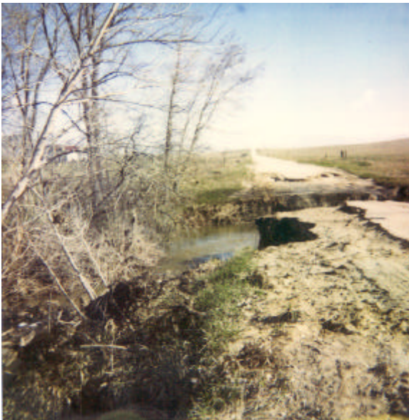
Washout caused by flooding of Big Sandy Creek on CR 149 near the town of Matheson.
