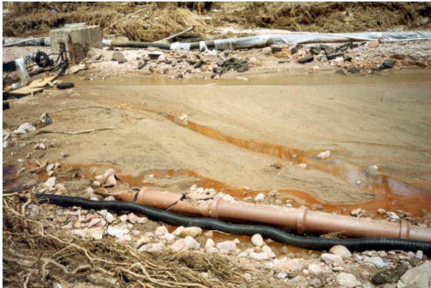
Damaged 16-inch non-potable water main in background and broken 12-inch sanitary sewer line in foreground. Area between I-25/Nevada Street off ramp and Colorado Avenue.
