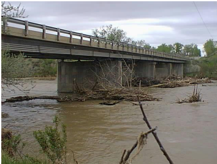
C-233 (Baxter Bridge) at Arkansas River showing debris accumulation on the west side of the bridge.
