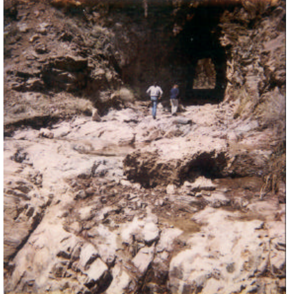
Damage to County Road 67, Phantom Canyon.
