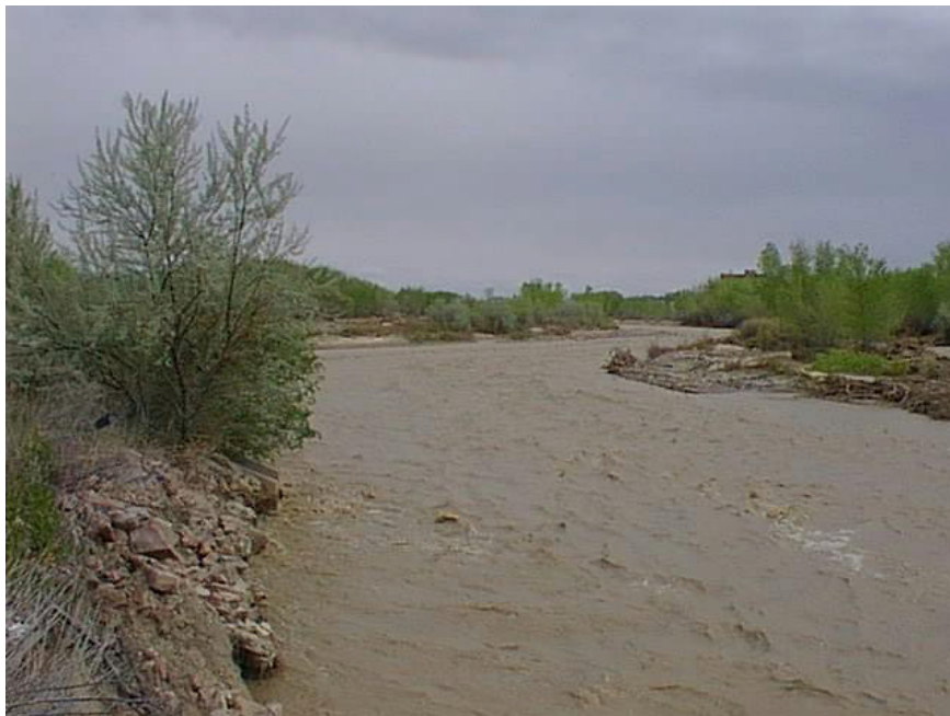
13 th Street at Fountain Creek looking upstream (riprap washed away from west bank).
