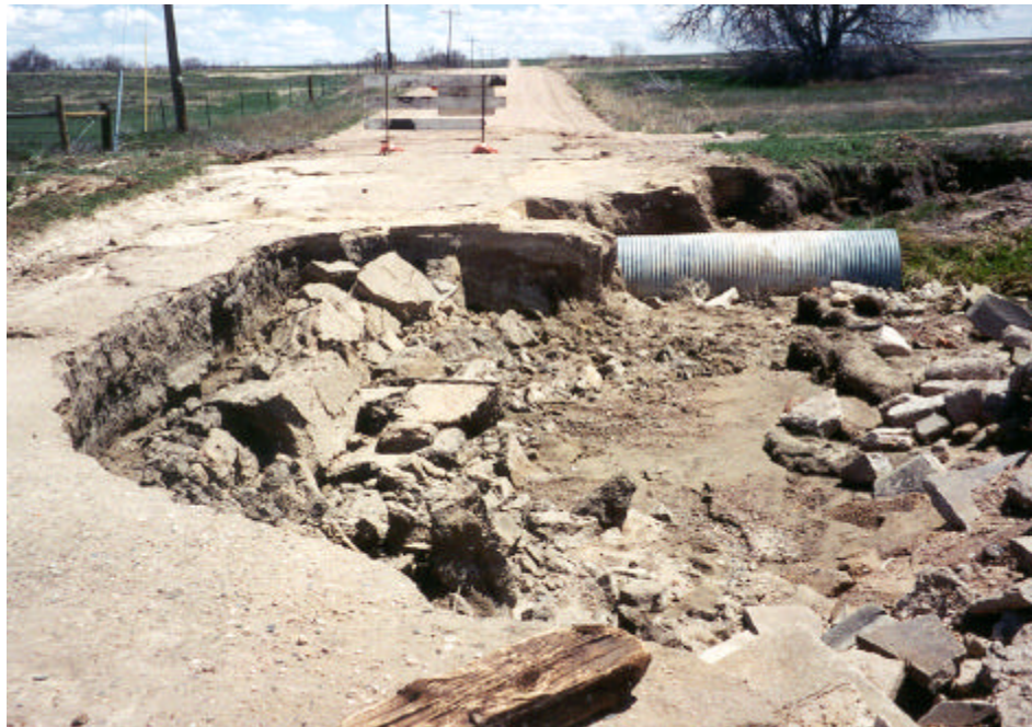
Scour hole approximately 80' L × 25' W × 3' D left by Owl Creek floodwaters on WCR 86 between WCR 45 and 49.
