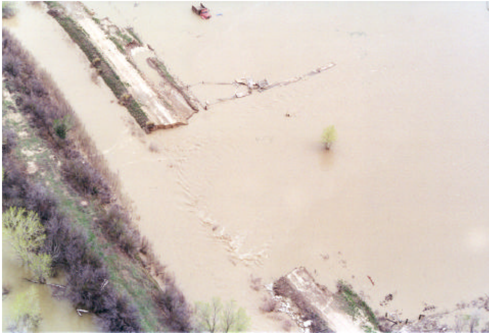
Overhead view of the break in the Fort Lyon Sluice #2 in North La Junta. May 3, 1999
