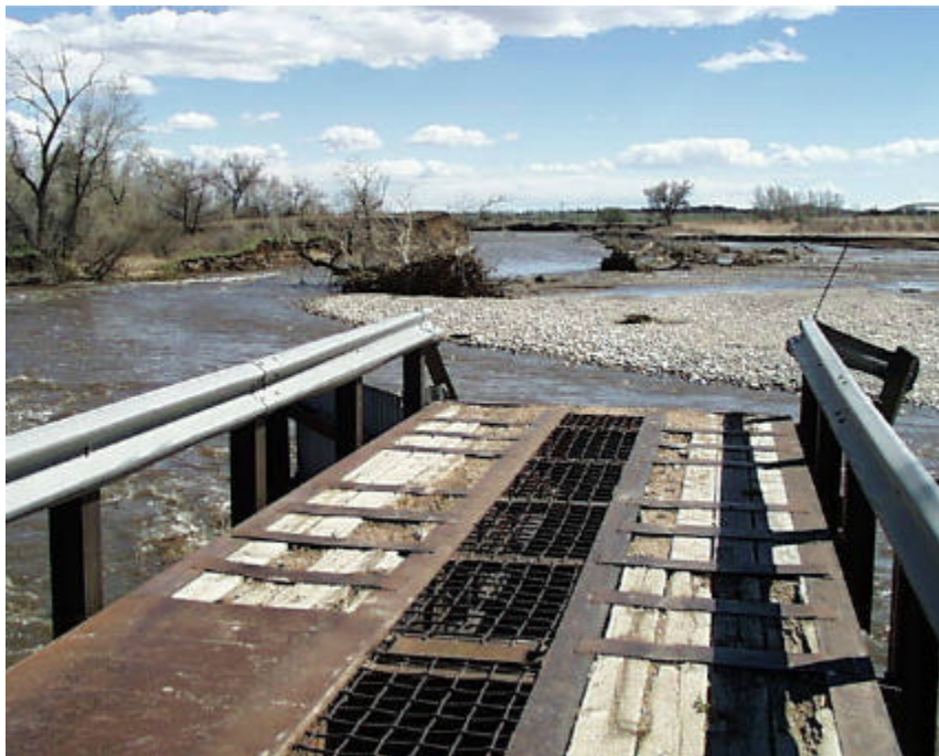
Haul Road bridge washout on Poudre River Bend near Boxelder Gage. May 4, 1999
