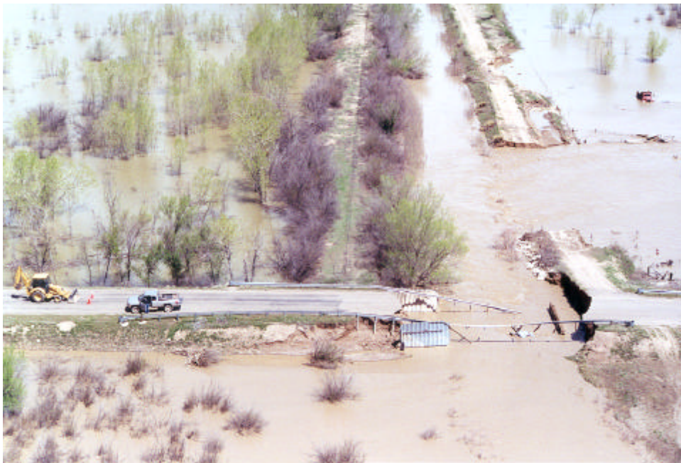
Washout of bridge along Dike Road and a break in the Fort Lyon Sluice #2 in North La Junta. May 3, 1999
