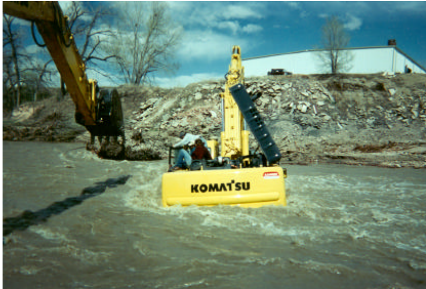
Emergency operations in Fountain Creek to repair 30-inch sanitary sewer break east of I-25 and north of Highway 85.
