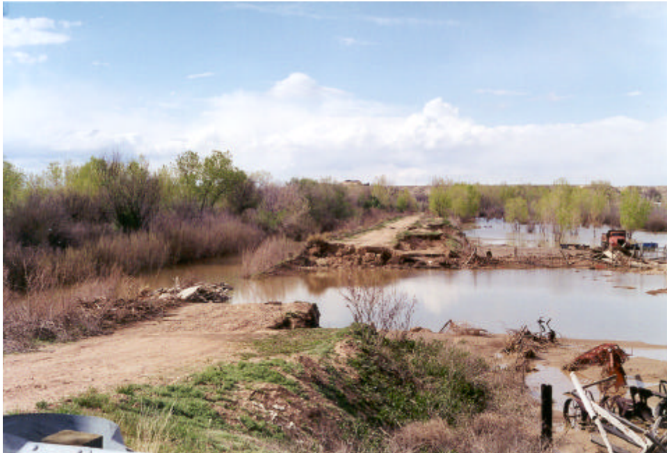
Break in the Fort Lyon Sluice #2 near Dike Road. May 5, 1999
