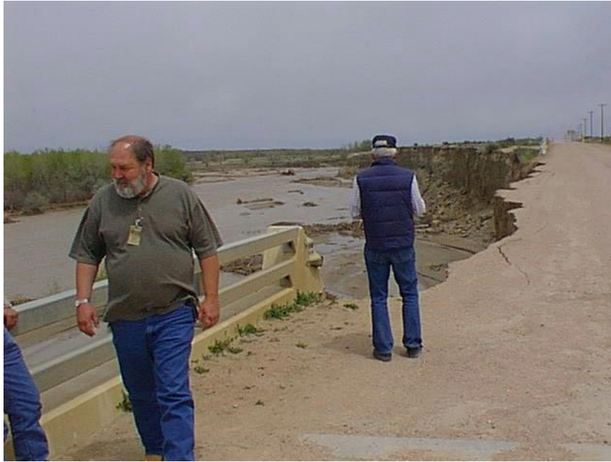
Erosion damage to Overton Road Bridge along Fountain Creek.
