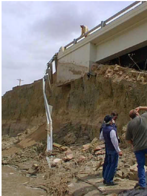
Erosion damage to Overton Road Bridge along Fountain Creek.
