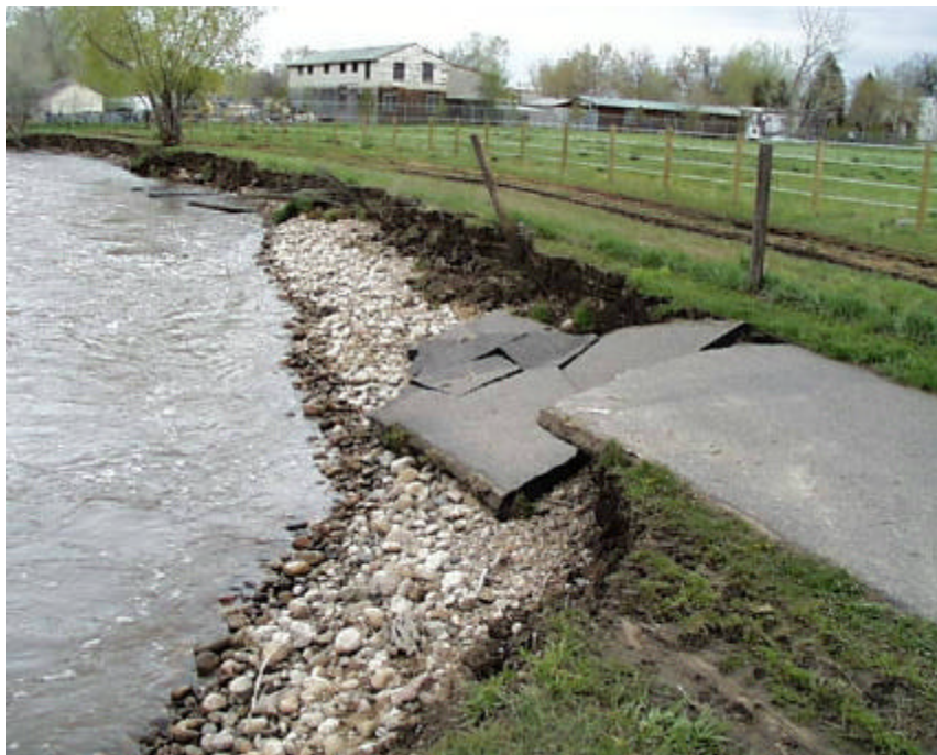
Damage by Poudre River to bike path near Shields Street in Fort Collins.
