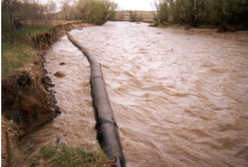
Erosion along Fountain Creek exposed a 30-inch sanitary sewer south of Circle Drive but did not cause a break.
