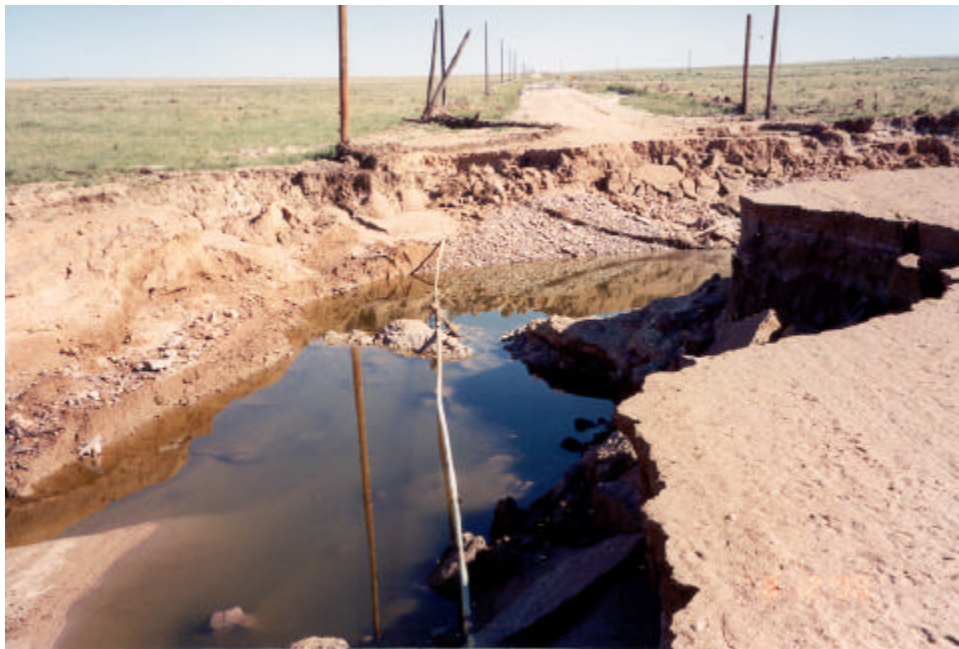
Wash out on Lane 21 at a second location showing exposed gas line (white conduit in middle of photo).
