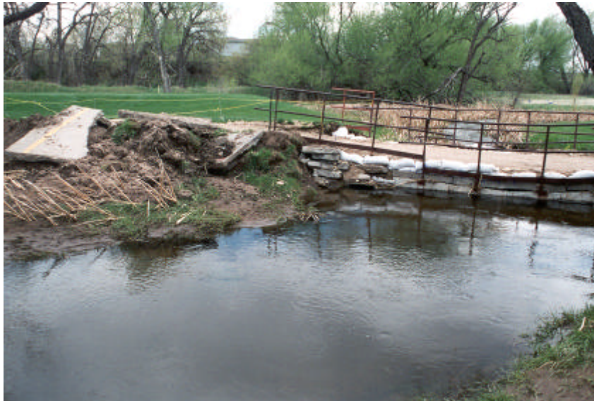
Temporary repair to cart path at the Mariana Butte Golf Course in Loveland.
