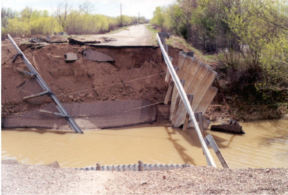
Dike Road bridge washout in North La Junta. May 5, 1999
