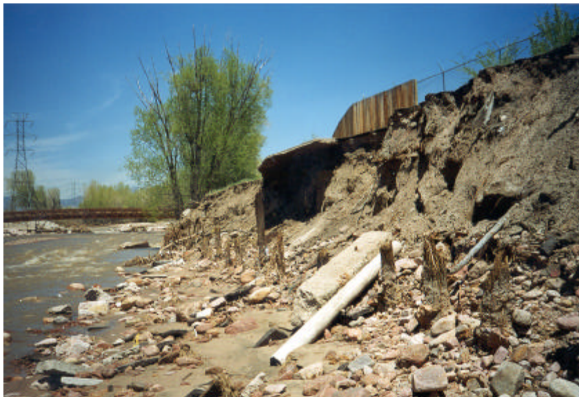
Fountain Creek erosion adjacent to the Las Vegas Street Wastewater Treatment Plant.
