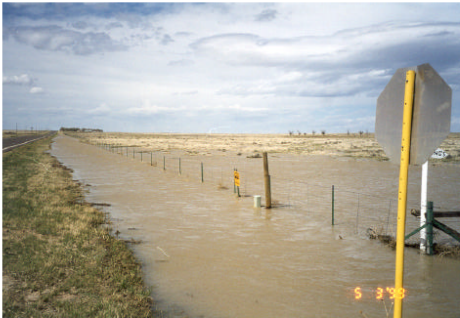
Drainage water fills borrow ditch along Highway 71.
