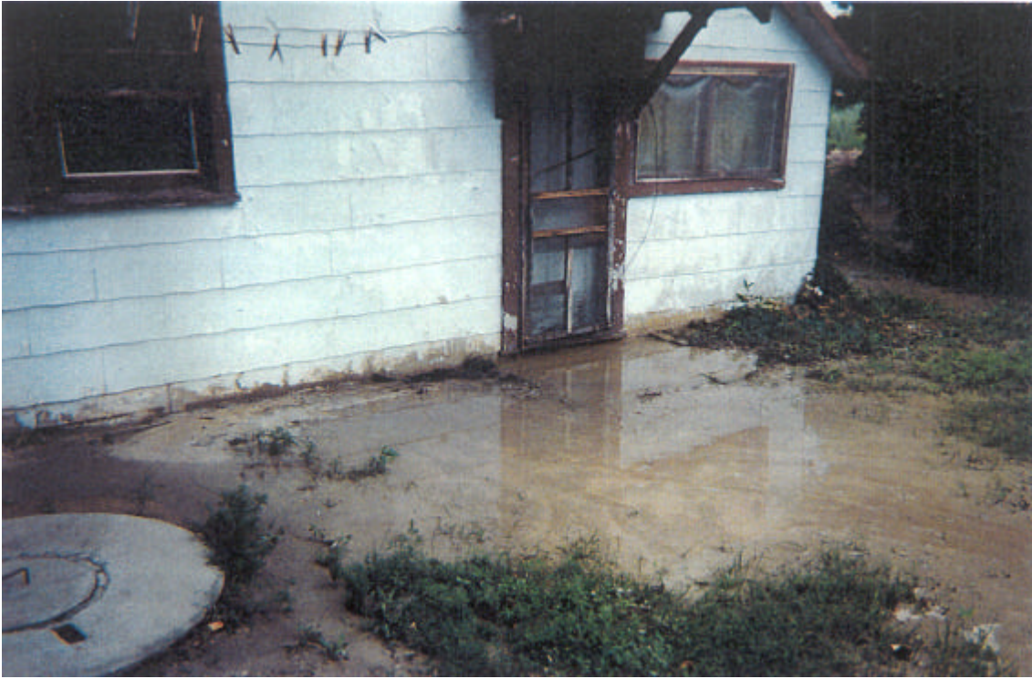
High water mark on house (August 11, 1999).
