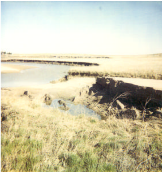
CR 118 east end washed out by flood waters in Big Sandy Creek.
