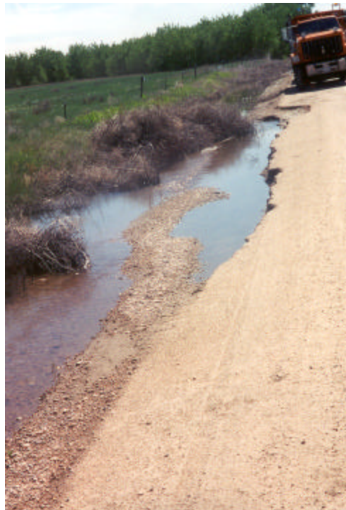
Shoulder erosion on WCR 74 from Crow Creek floodwaters between WCR 392 and 79.
