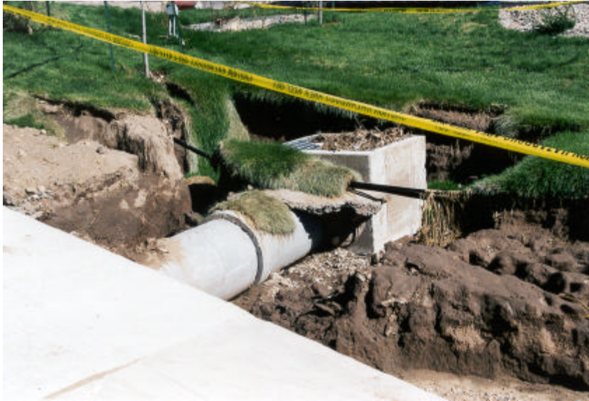
Erosion damage to storm drain inlet at Highway 287 and the Big Thompson River in Loveland.
