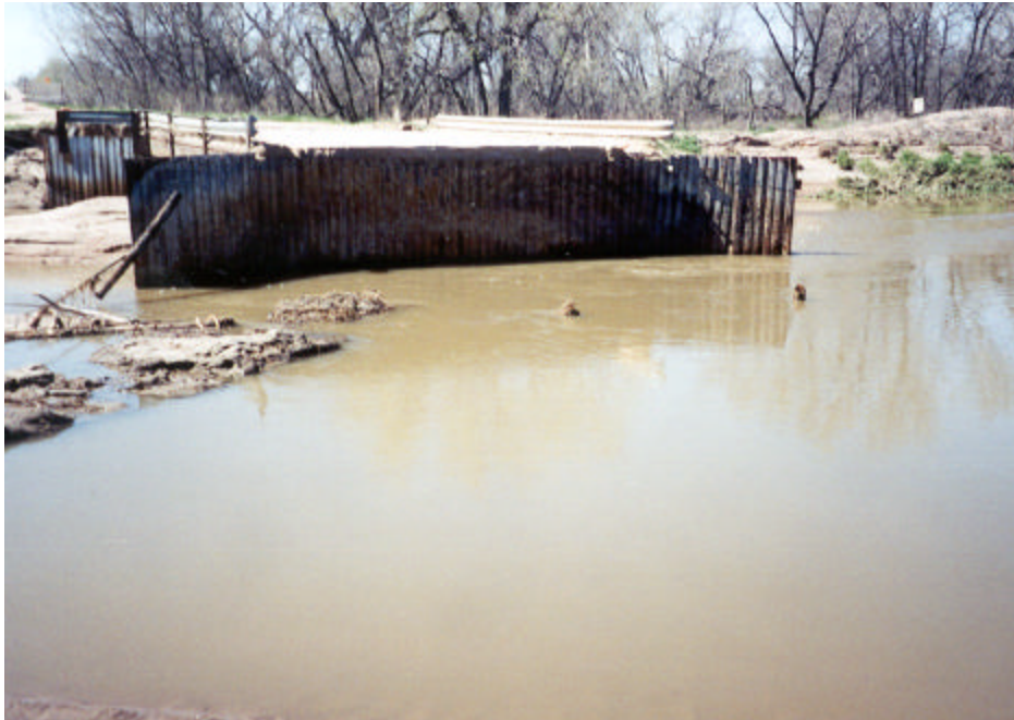
WCR 87 crossing of the Poudre River between WCR 42.5 and 44.5 where floodwaters washed out both approaches to the crossing.
