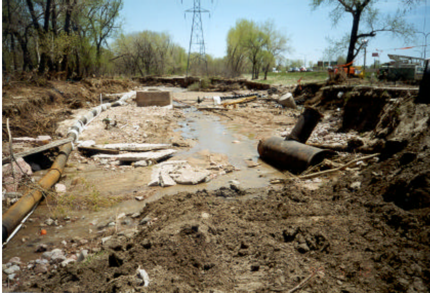
Erosion damage by Fountain Creek to 2,300 feet of 16-inch DIP non-potable water main between I-25/Nevada Street off ramp and Colorado Avenue.
