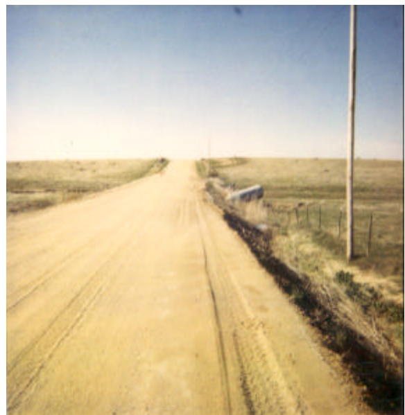
48-inch diameter culvert bent upward by fast flowing flood water from Middle Rush Creek, 2 miles south of CR 66 on CR 149.
