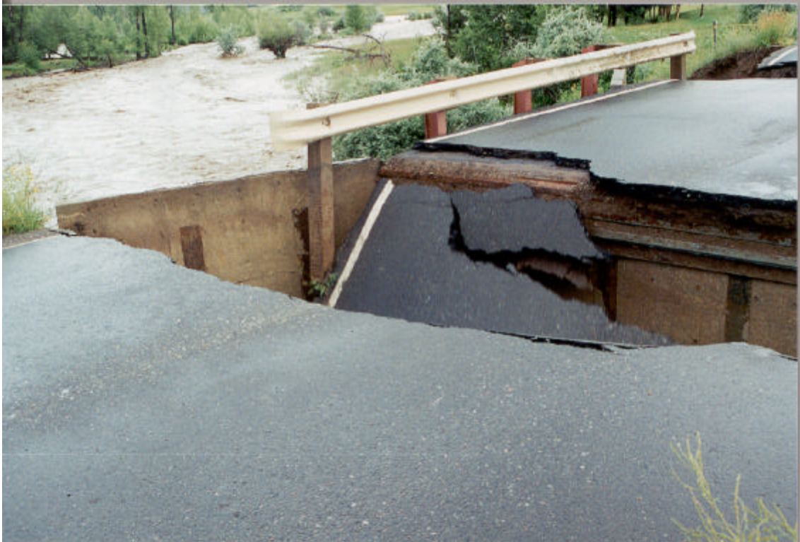
Destroyed County Road 24A bridge across Dallas Creek.
