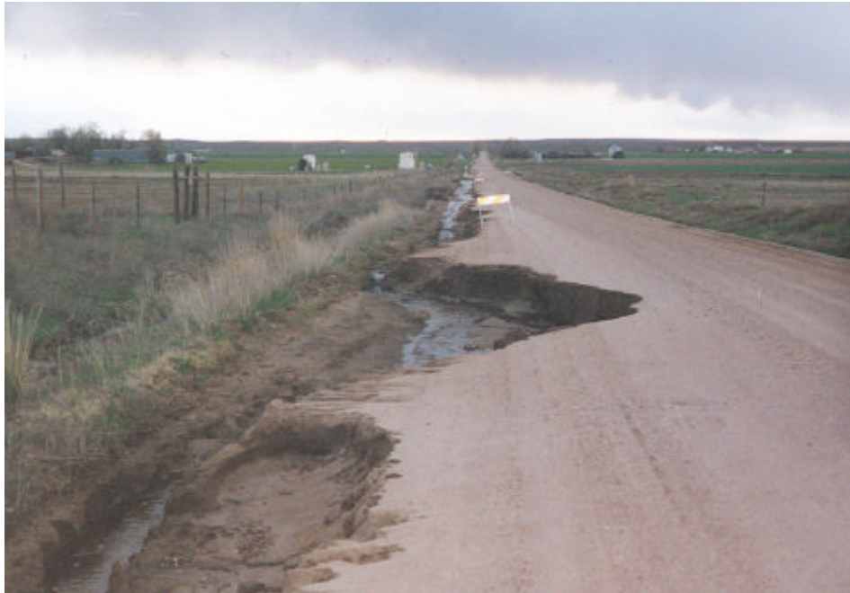
Erosion damage by local runoff to WCR 36 between WCR 49 and 53.
