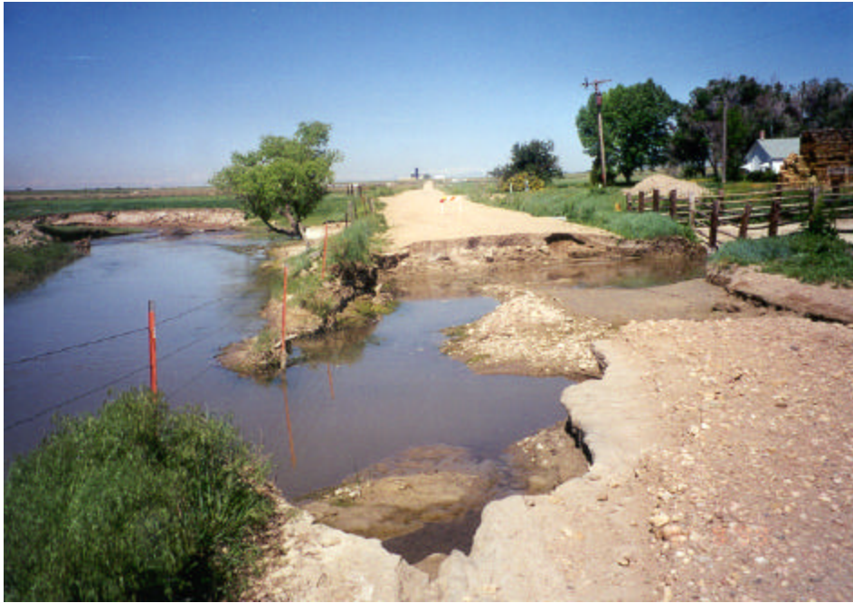
Erosion damage to WCR 64 from Crow Creek floodwaters between WCR 57 and 59.
