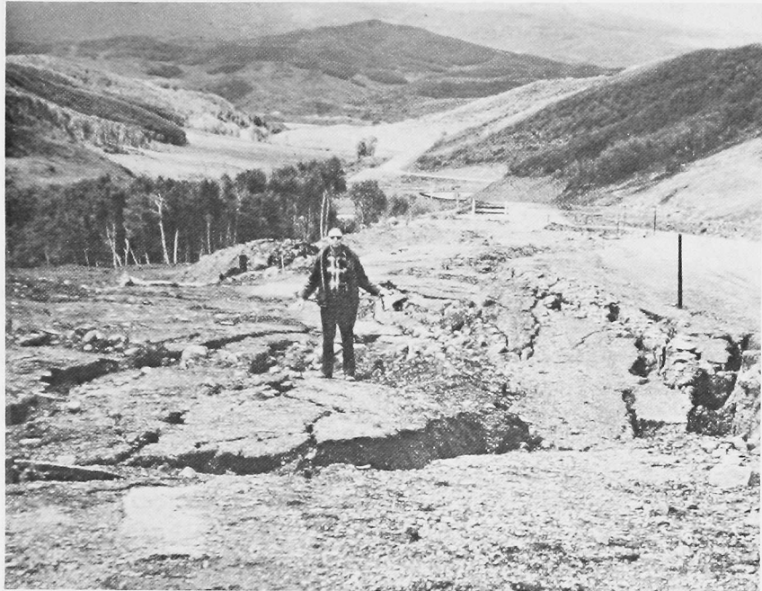
Figure 11. THIS HIGHWAY, BUILT IN A HIGHLY UNSTABLE AREA, WAS SEVERELY DAMAGED BY A LANDSLIDE.
