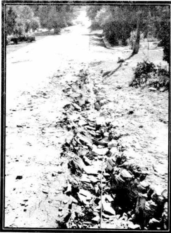
This was one of many roads in town that suffered erosional damage from flood waters.
