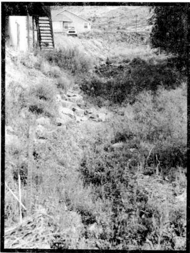
The northern section of the drainage ditch overgrown with vegetation.
