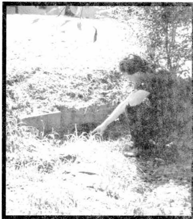
Underground drainage pipe filled with sediment and debris.
